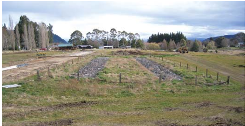
Denitrification beds at Kinloch filled with sawdust and bark. These beds remove nearly all the nitrogen from wastewater passing through them
